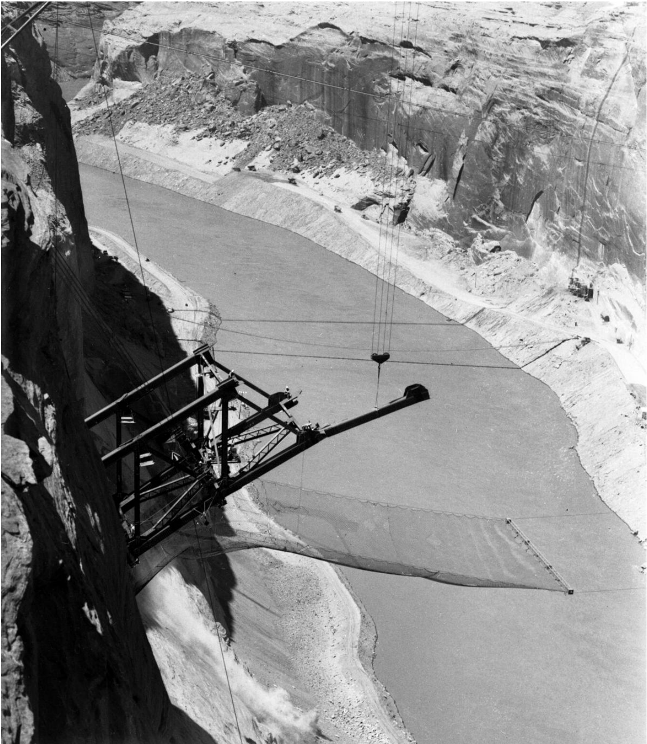
Steelworkers sit on the steel span for Glen Canyon bridge under construction high above the Colorado River in the late 1950s.
