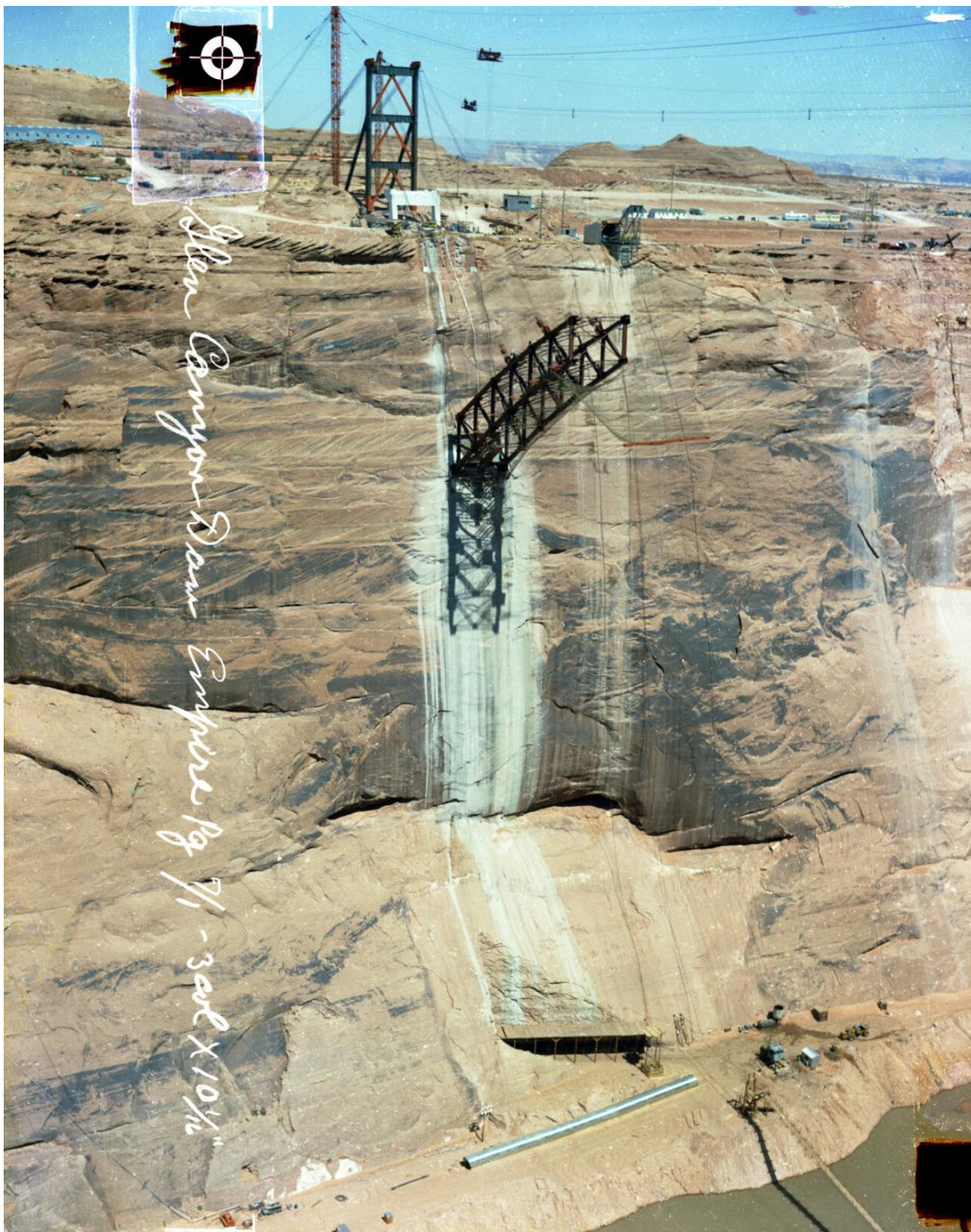
The bridge span emerges from the anchorage in the wall of Glen Canyon just west of the dam site under construction, late 1950s.
