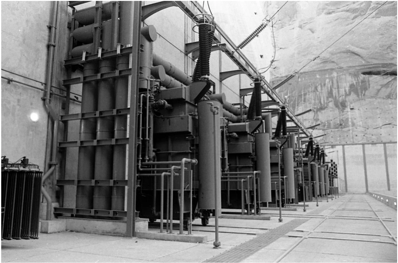
The transformer complex during the official dedication of Glen Canyon Dam near Page, Ariz. on Sept. 22, 1966.
