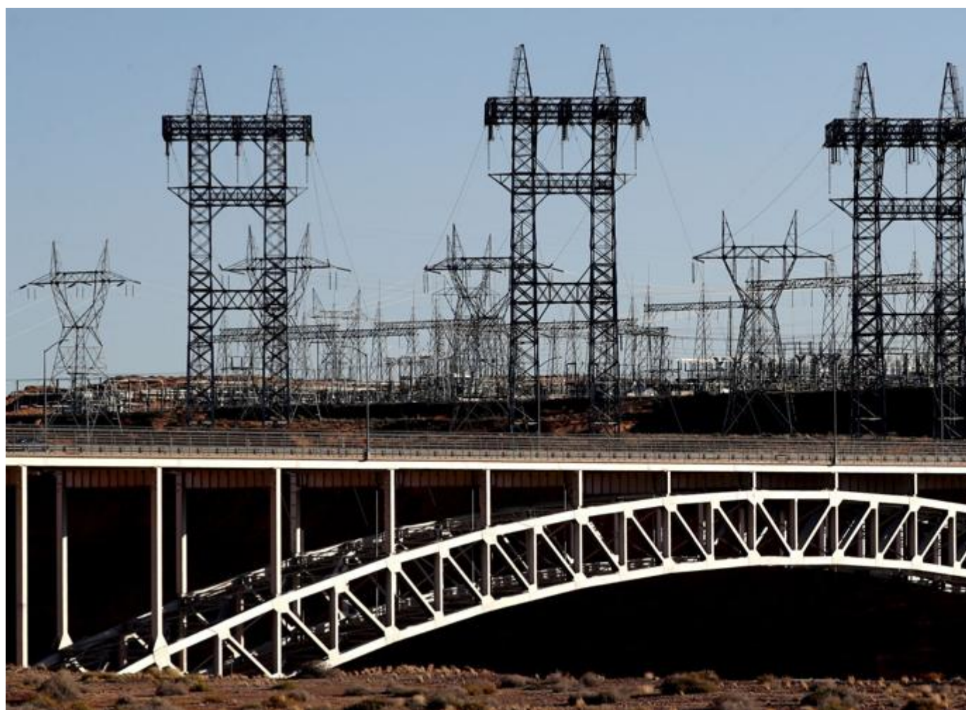
The electrical substation fed by hydroelectric turbines inside Glen Canyon Dam shown beyond Glen Canyon Dam, Kelly Presnell, Arizona Daily Star
