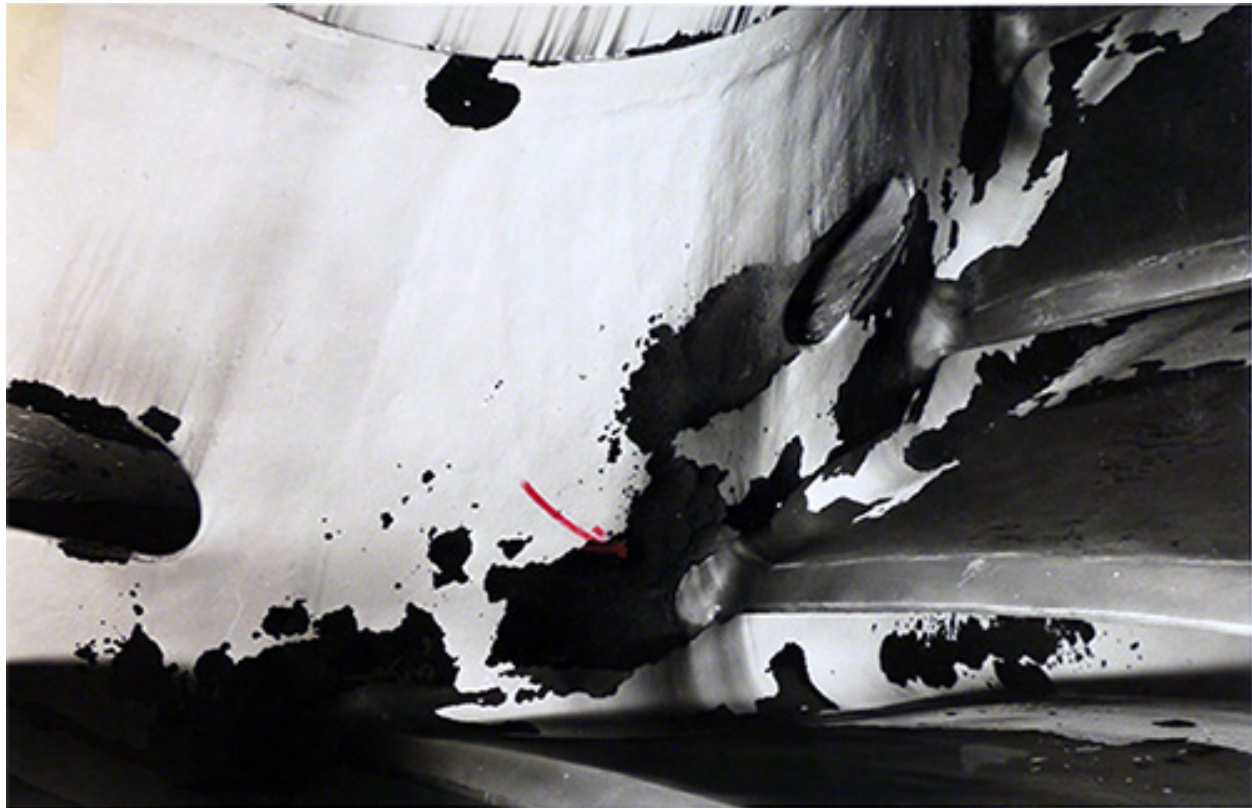
P 557-420-10576 Glen Canyon Unit--C.R.S.P. NA Unit 2. Looking at the upper end of the trailing edge of 3 of the 15 buckets of the runner. Arrow points to a spot on the crown which had cavitated deeply enough to cause Mr. Claude Tate, the erecting engineer, to have it gouged to 7/8-inch depth and filled with stainless steel electrodes. Contractor: Baldwin-Lima-Hamilton Corp., Contract No. 14-06-D-3506. Invitation No. DS-5234. 2-17-65 F. Finch
