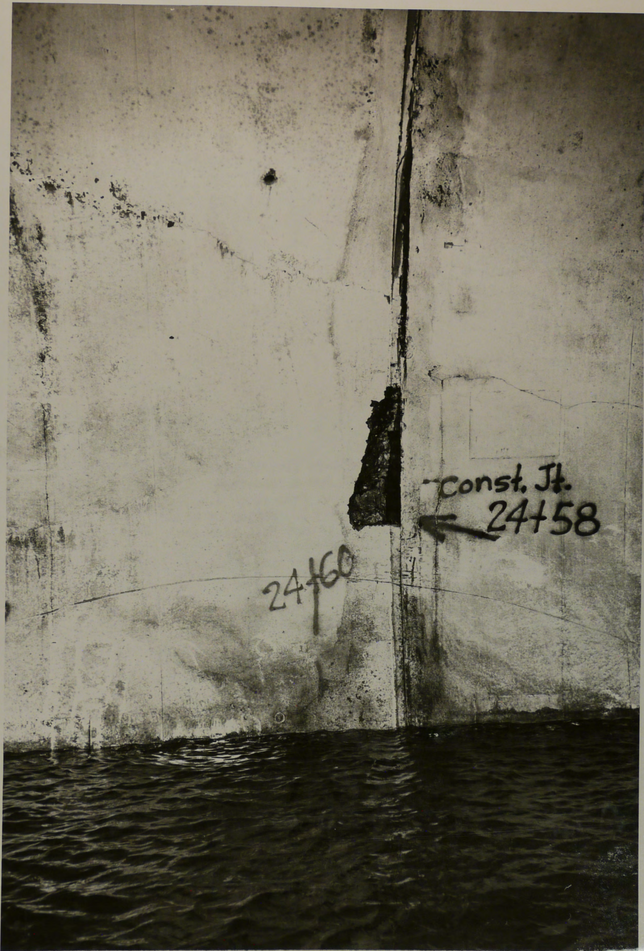
P 557-420-10795 Glen Canyon Unit--C.R.S.P. NA Hole in concrete lining of left diversion tunnel 3-23-65
