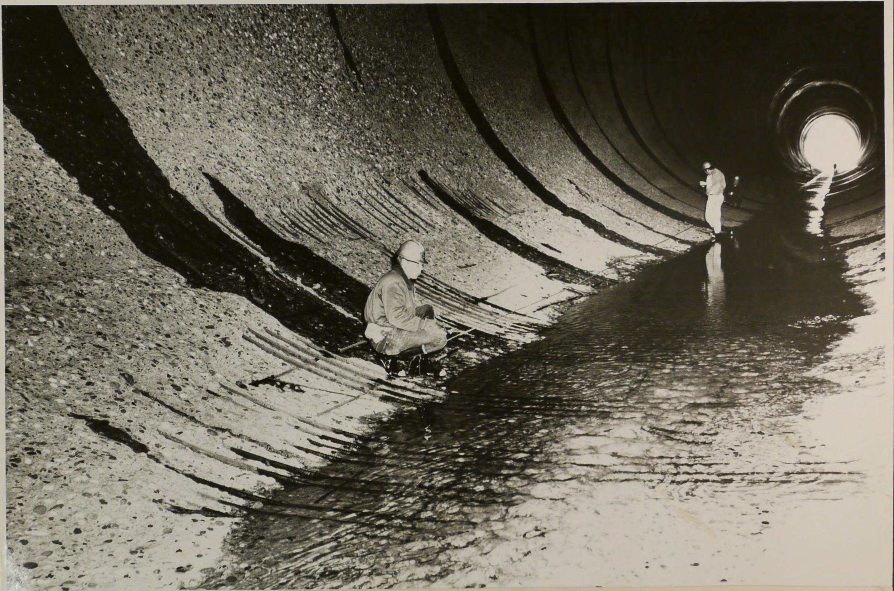
P 557-420-10602 Glen Canyon Unit--C.R.S.P. NA View of left spillway tunnel below ; the outlet gates showing erosion caused by heavy discharges. Contractor: Merritt-Chapman and Scott Corp., Contract No. 14-06-D-2403. Specs. No. DS-4825. 2-24-65 F. Finch
