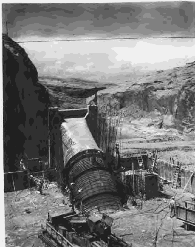
Figure 271.—Forms and reinforcement steel for the penstock transition concrete and trashracks being installed in block 16 on penstock 2. P557-420-7365, July 27, 1962.
