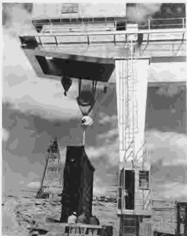
Figure 274.—Gantry crane lowering 120-ton fixed-wheel gate into the tracks of penstock No. 8. P557-420-9711, April 20, 1964.
