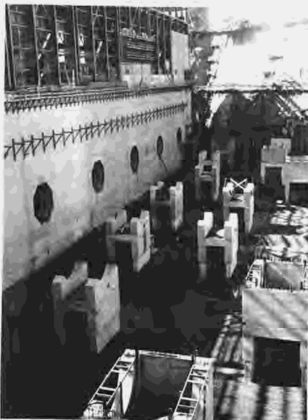
Figure 283.—Aggregate backfill placed between dam and powerplant. Trenches are excavated between penstock piers for tile drain pipe. P557-420-6773, February 21, 1962.
