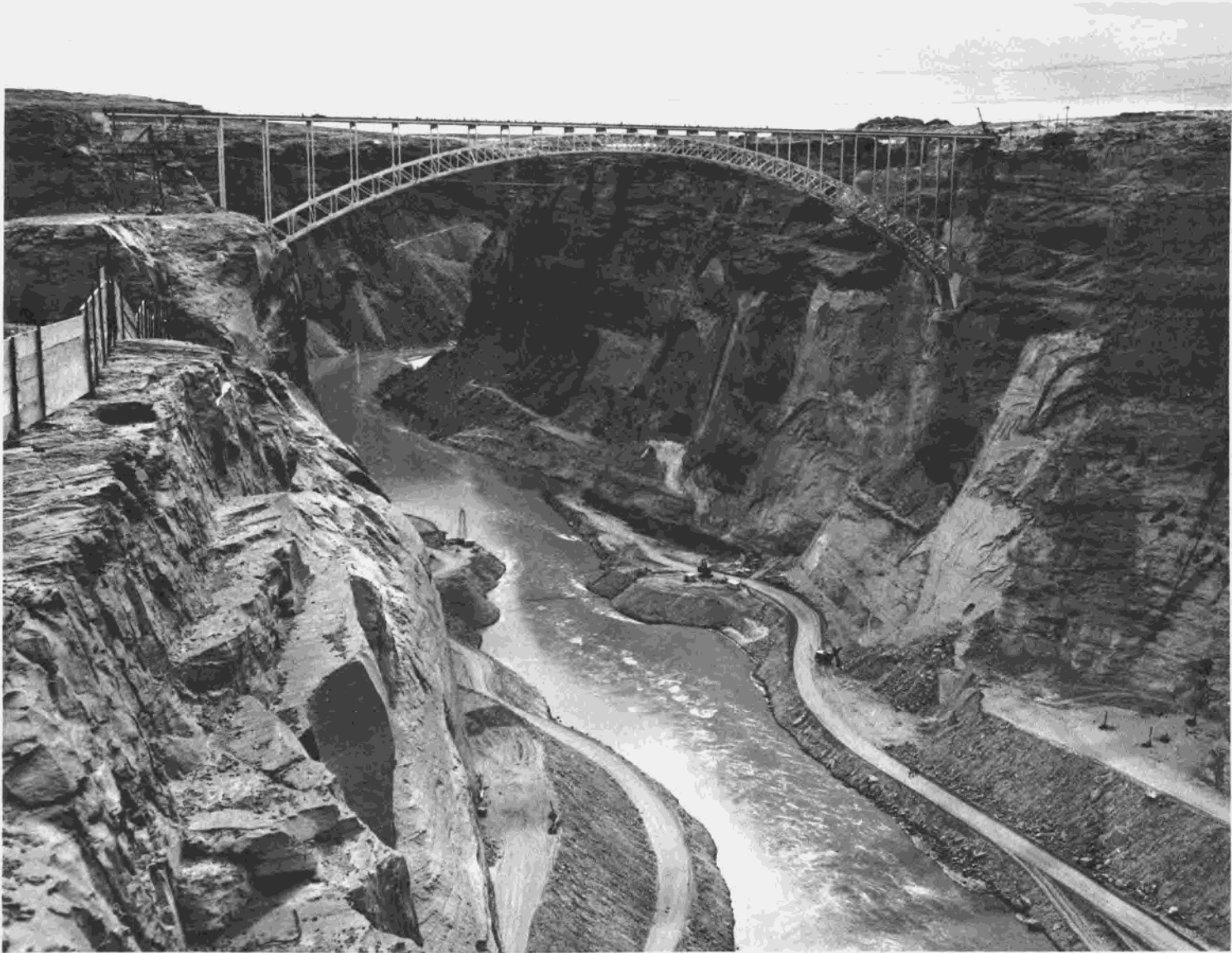
Figure 2.—View downstream showing the nearly completed Glen Canyon Bridge, the downstream cofferdam, and the right keyway. P557-400-236, January 30, 1959.
