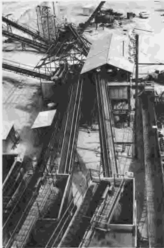
Figure 256.—Heavy-media separation plant (center) at Wahweap aggregate plant. Separator for No. 8 to No. 4 sand is on the left and separator for 3/4- to 1-1/2-inch aggregate and No. 4 to 3/4-inch aggregate is on the right. Raw feed bins are at bottom. Raw feed belts to plants are at center. Waste conveyor is at the right. At top left is screening plant for separation of No. 4 to 3/4-inch and 3/4- to 1-1/2-inch beneficiated aggregate. At top center rod mill is being erected for production of sandblast sand. P557-420-4609, March 25, 1960.
