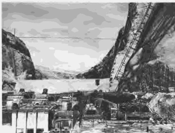
Figure 276.—View of construction operations in the powerplant and dam from the downstream cofferdam. Sections of outlet pipes 3 and 4 are in place in the machine shop bay above pipes 1 and 2 (right foreground). P557-420-5819, March 23, 1961.
