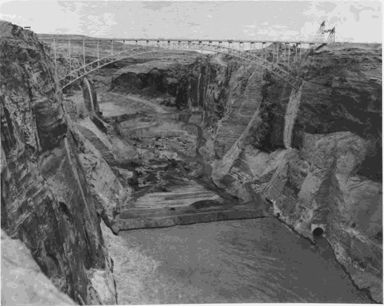
Figure 253.—Glen Canyon damsite as seen from progress photo point No. 1, approximately one-half mile downstream from the damsite on the west rim of the canyon. Note the heavy equipment working on the keyway foundation. P557-420-3817, May 20, 1959.
