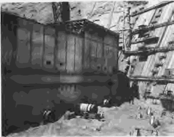
Figure 284.—Construction view of upstream face of powerplant and downstream face of dam. Note penstock installation from powerplant to dam. P557-420-7116, June 7, 1962.
