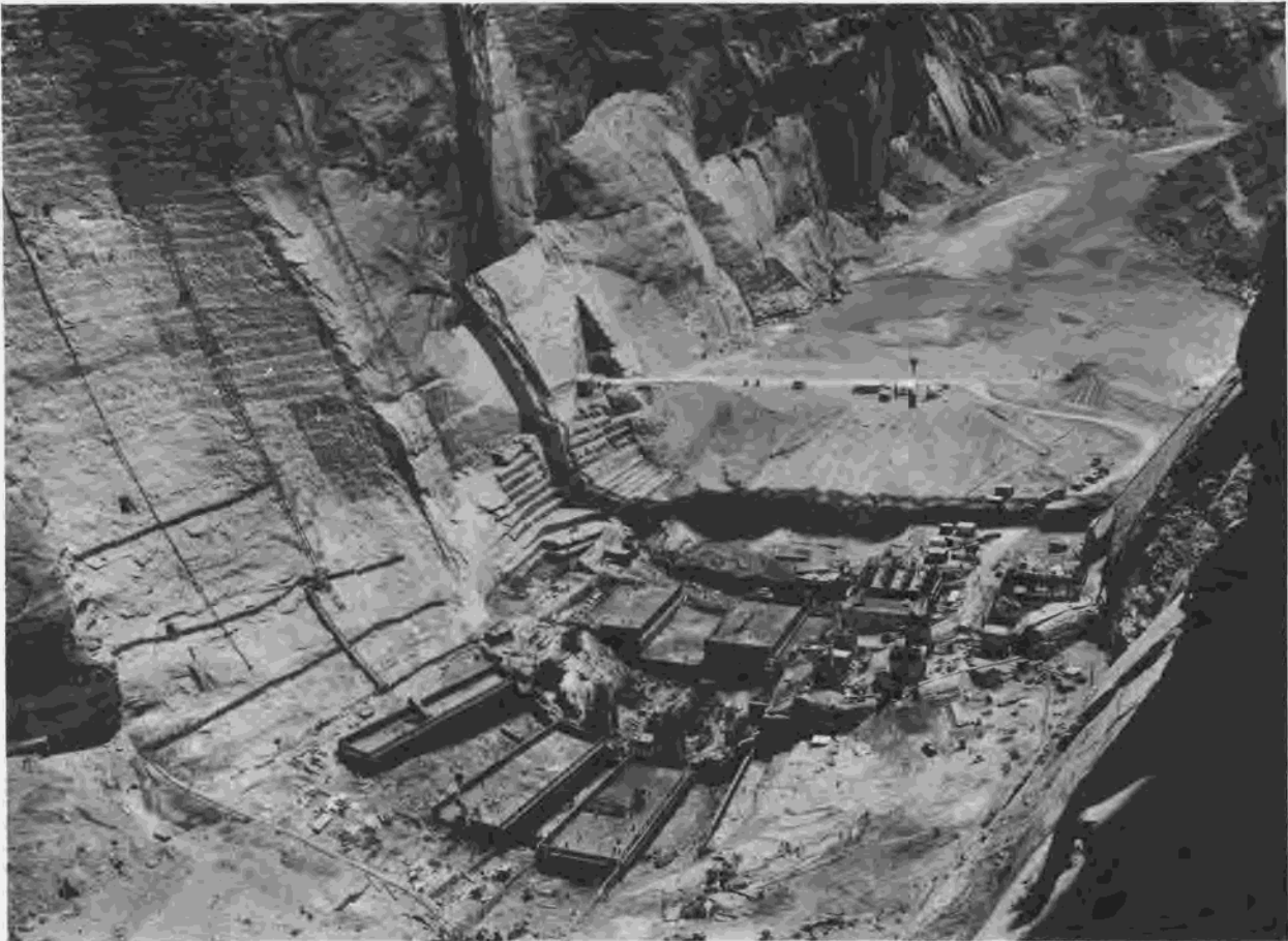
Figure 254.—View downstream from right spillway showing concrete blocks rising in dam and powerplant area. P557-420-5165, August 4, 1960.
