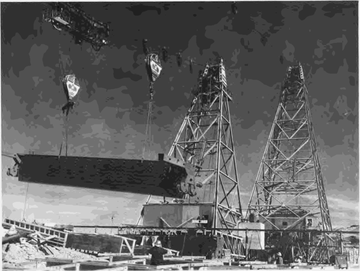
Figure 261.—A 44-ton section of the crane for the powerplant is hoisted into the air by both of the 50-ton-capacity cableways. Both cableways were used because of the awkward length of the section. P557-420-6678, February 4, 1962.
