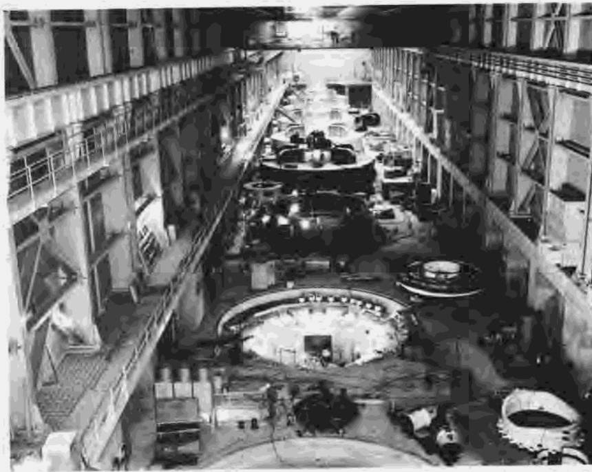
Figure 289.—Interior of powerplant during generator installation, as seen from the service bay. P557-420-10488, January 27, 1965.
