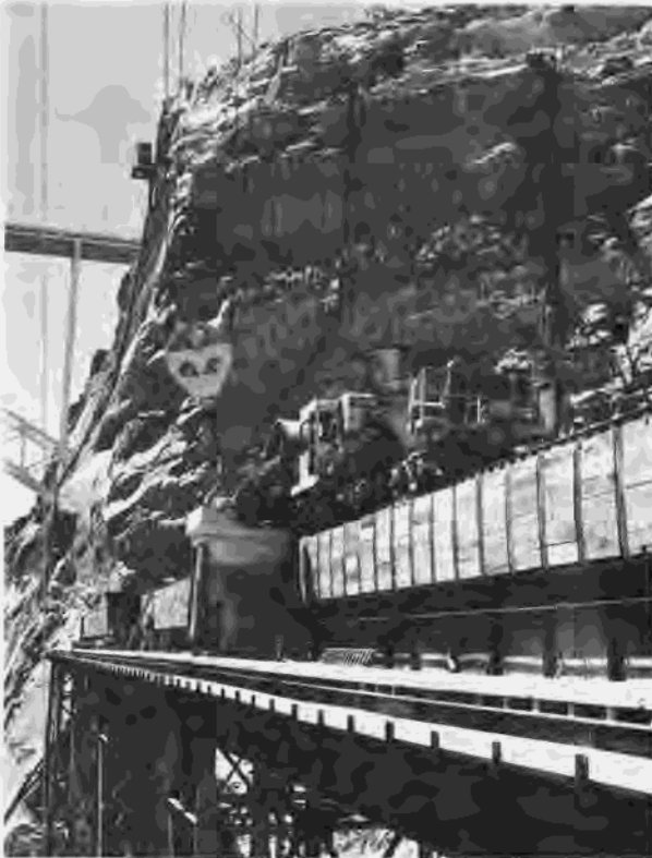
Figure 264.—Transfer ladle car dumping its load of concrete into a 12-cubic-yard bucket high over the Glen Canyon damsite. Note abutment of Glen Canyon Bridge in background. P557-420-5057, July 11, 1960.
