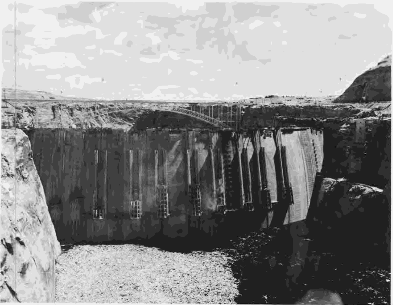
Figure 266.—Upstream face of Glen Canyon Dam during construction as seen from the footbridge. P557-420-8625, July 25, 1963.
