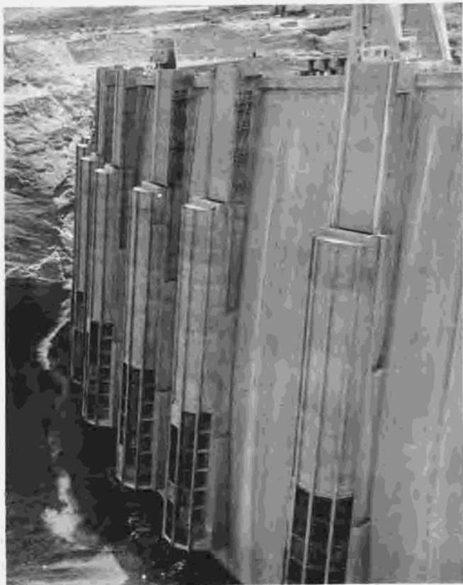
Figure 270.—View of upstream face of Glen Canyon Dam showing trashrack construction. Trashrack structure No. 8 is in foreground. P557-420-9794NA, May 27, 1964.
