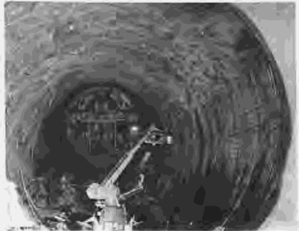
Figure 252.—Installing reinforcing bars in elbow section of left spillway. Slipform is in background. P557-420-12375, June 14, 1966.
