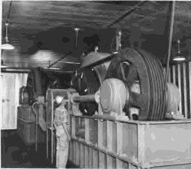
Figure 262.—Interior view of the hoist room in the huge head tower of the mobile cableway. P557-420-4818, May 1960.
