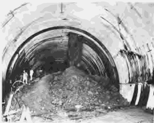
Figure 250.—View looking upstream to plug section in left diversion tunnel. Sand and rock are falling through holes from elbow excavation above. P-557-420-11896, February 9, 1966.
