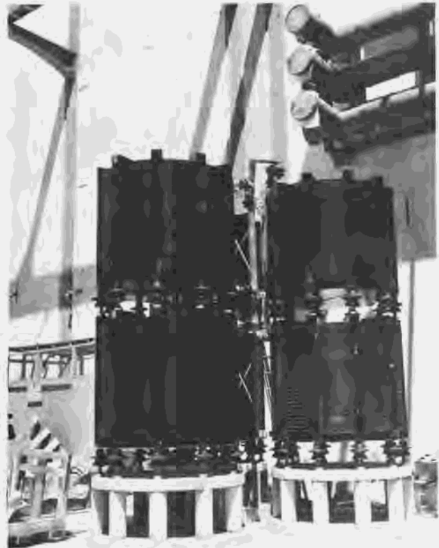
Figure 292.—Closeup view of two shunt reactors. P557-420-9943, July 13, 1964.
