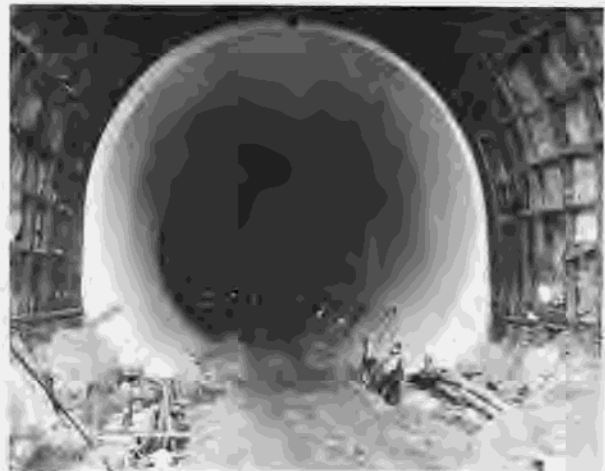
Figure 249.—View of north portal of the right diversion tunnel showing concrete lining in place. P557-420-2818, September 17, 1958.
