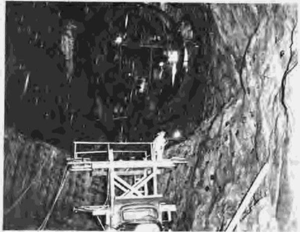
Figure 251.—Looking up in elbow section of left spillway. Drillers at work in foreground. P557-420-11982, February 23, 1966.
