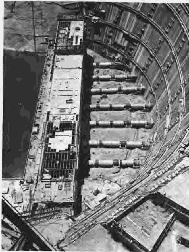
Figure 269.—View looking down on Glen Canyon Dam and Powerplant. Note penstock installation between dam and powerplant. P557-420-7212, July 5, 1962.
