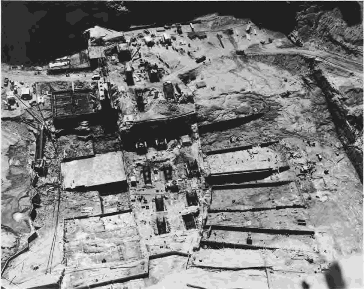
Figure 263.—View looking down on the damsite from the canyon rim. Powerhouse is at left, dam at right, with penstock foundations between them at center. P557-420-5038, July 7, 1960.
