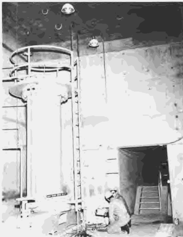
Figure 275.—General view of equipment used in testing of river outlet No. 4 at various flow conditions. Test station is located in the ring-follower gate chamber in dam block 5 at elevation 3387.5. P557-420-11016, May 24, 1965.
