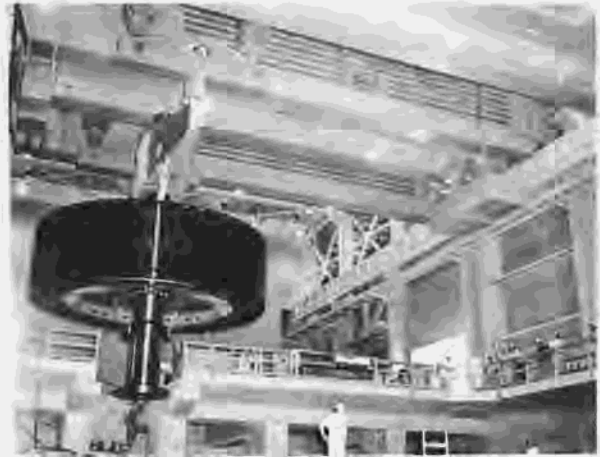
Figure 290.—Two 300-ton cranes with lifting beam moving unit 8 rotor from assembly pad to final placement location. P557-420-11333, July 21, 1965.
