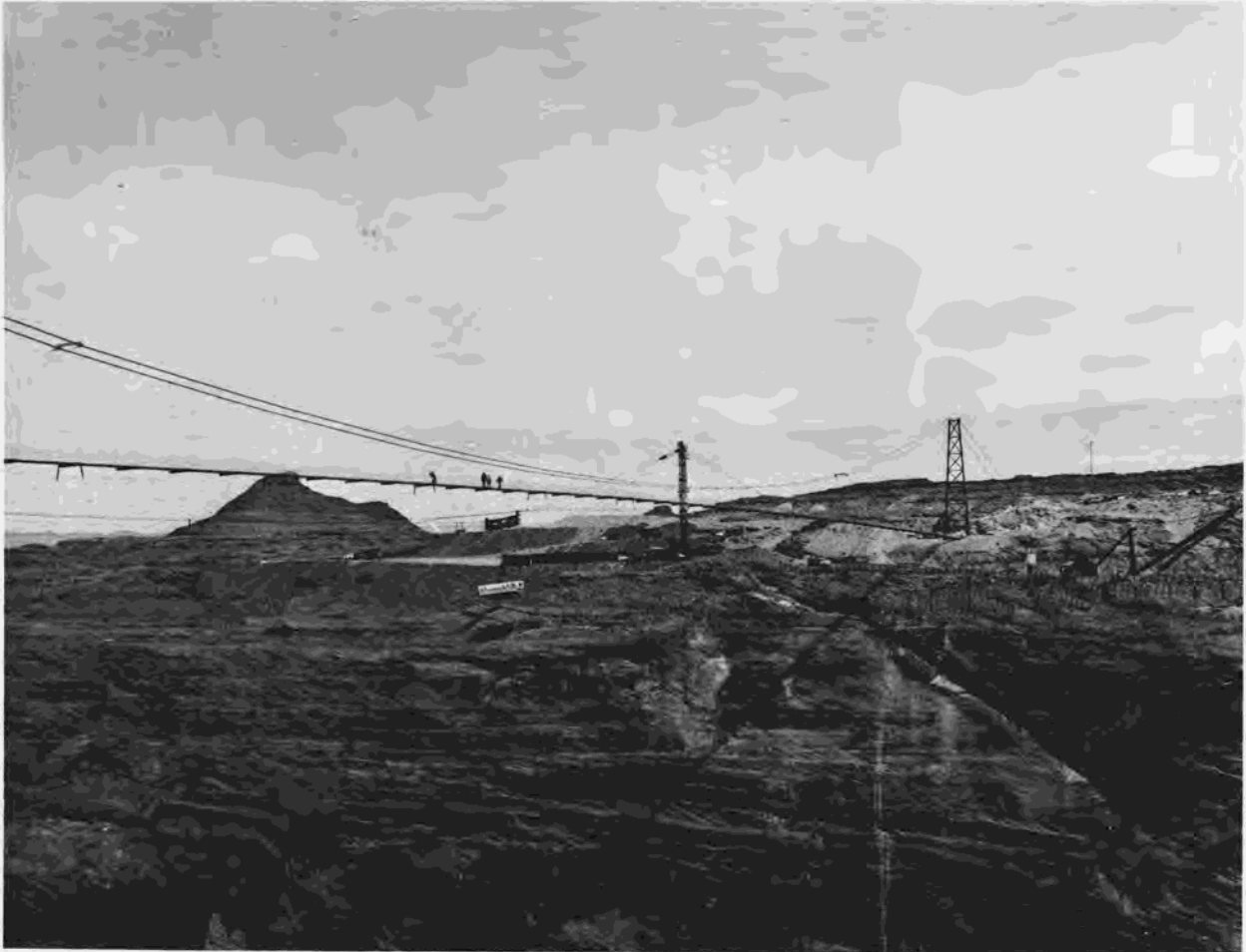
Figure 247.—View of prime contractor's highline cableway being used to move trailers from west side to east side of the Colorado River. Footbridge is in foreground of trailer being taken across. P557-420-1721, February 14, 1958.
