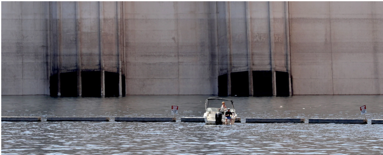
A small fishing boat ties up on the breakwater just outside the intakes for the Glen Canyon Dam, Glen Canyon National Recreation Area, Page, Ariz.. The penstocks (water intakes to the power turbines) are revealed for the first time since 1967 when the Lake Powell was being filled. Kelly Presnell Arizona Daily Star
