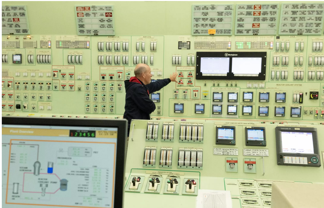
License instructor Dan Stermer gives a tour of a simulated control room identical to the actual control room at Diablo Canyon Power Plant on July 31. It's used to train operators and practice emergency response.
