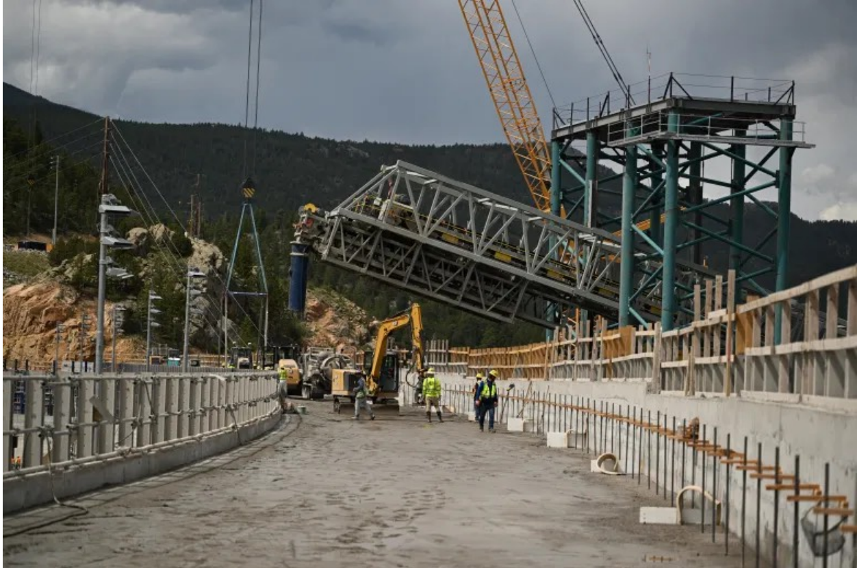
Photo caption: Work continues on the Denver Water Gross Dam project, on June 3, 2026, in Boulder County, Colorado. (Photo by RJ Sangosti/The Denver Post)
