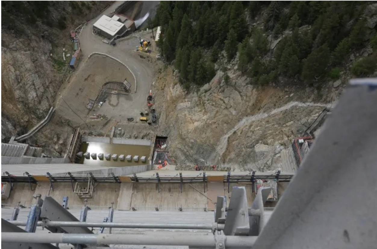
Photo caption: Denver Water's project crews near completion on the expansion of Gross Dam on June 3, 2026, in Boulder County, Colorado. (Photo by RJ Sangosti/The Denver Post)
