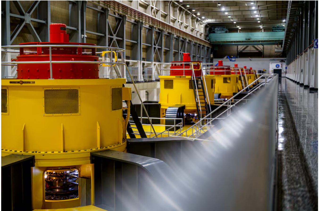
Photo caption: (Trent Nelson | The Salt Lake Tribune) Some of the eight generators at Glen Canyon Dam in Page, Ariz., on Tuesday, May 20, 2025.
