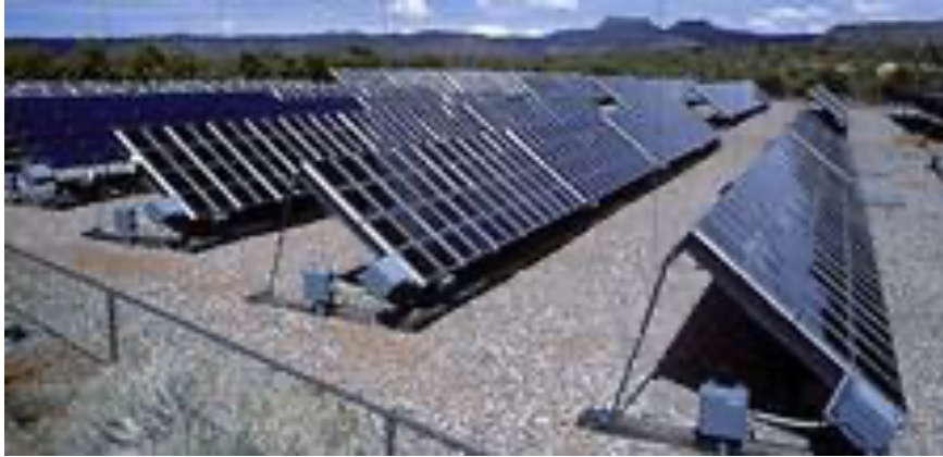
Solar array at Natural Bridges National Monument
